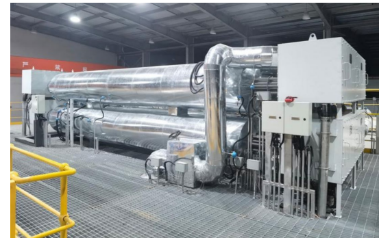
Cosin Solar's 6.3 kV high-temperature molten salt heater (Source: unpublished direct communication with Cosin).
