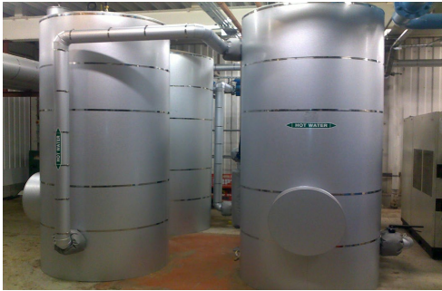
Hot water storage coupled to a heat pump system at the Nestle confectionery plant in Halifax, UK
