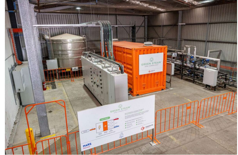
Graphite Energy Green Steam™ system at Mars Petcare Wodonga.
