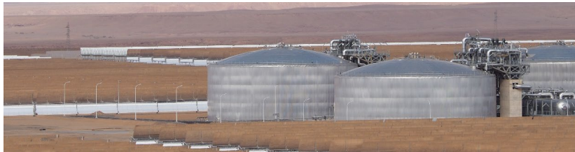
Two-tank molten salt storage at the Noor CSP plant, Morocco. Photo: Coventry
